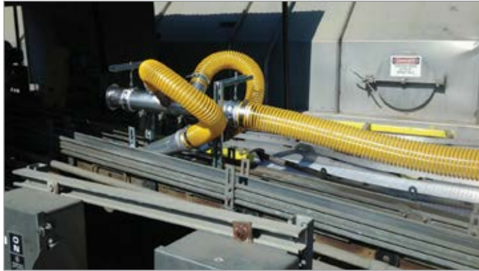
Image 3: Sample installation of an air delivery system from Process Air Solutions
