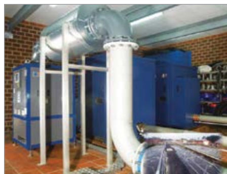
Figure 1 Aerzen AT turbo blower and two PD blowers processing air at a Bremervörde, Germany WWTP.
