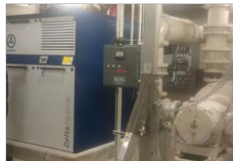
The City of Anacortes replaced a 125HP multistage centrifugal blower (right) with an Aerzen D 62S 75HP hybrid blower (left)
