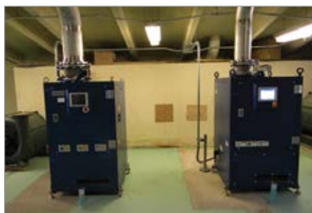
Aerzen TB100 turbo blowers at the Blue River Wastewater Treatment Plant (Silverthorne, Colo.)
