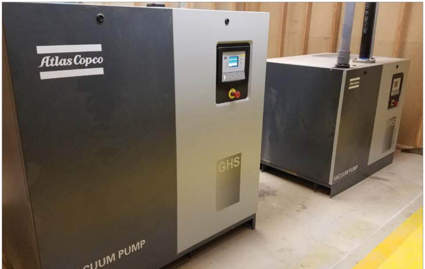
The centralized Atlas Copco models GHS 1300 VSD+ and one GHS 730 VSD+ minimize power draw during the vacuum off portion of the production cycle.
