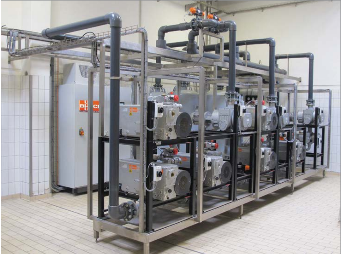
Figure 2: Busch centralized vacuum system at DMK in Georgsmarienhütte.
