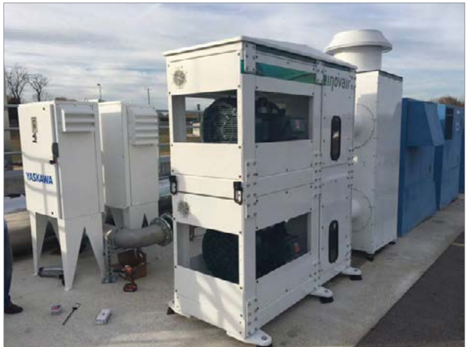
Figure 1: Shown is the Inovair IM prototype during installation. The customer-specified Variable Frequency Drives are visible in the background.
