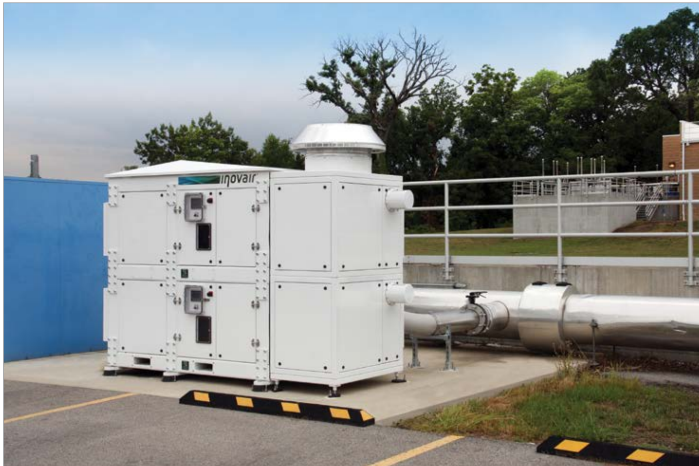
The IM unit on Basin 3 offers a more compact footprint and increased weather resistance compared to the prototype IM blower on Basin 2. Plant operators appreciate the sound level of less than 82 dBA.
