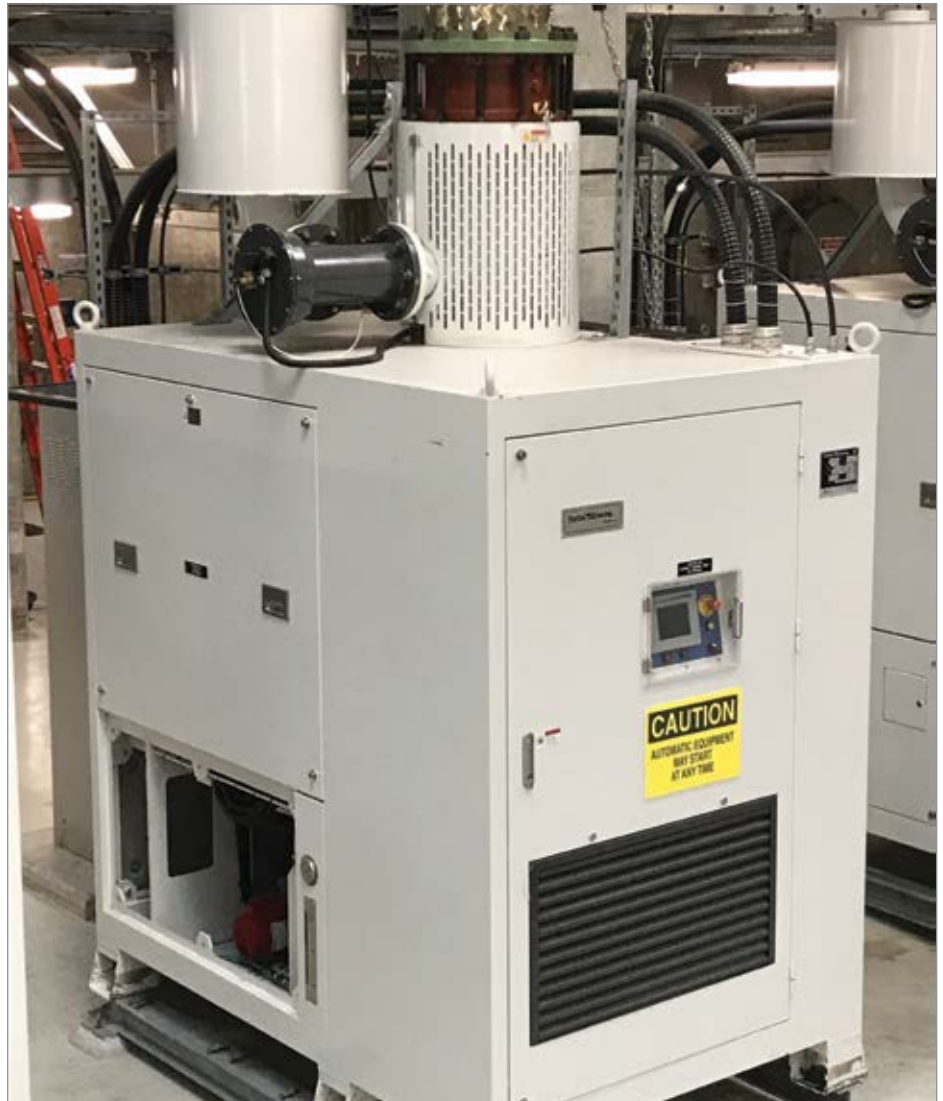
Aeration blowers continue to play an important role in helping treatment plants achieve energy savings.
