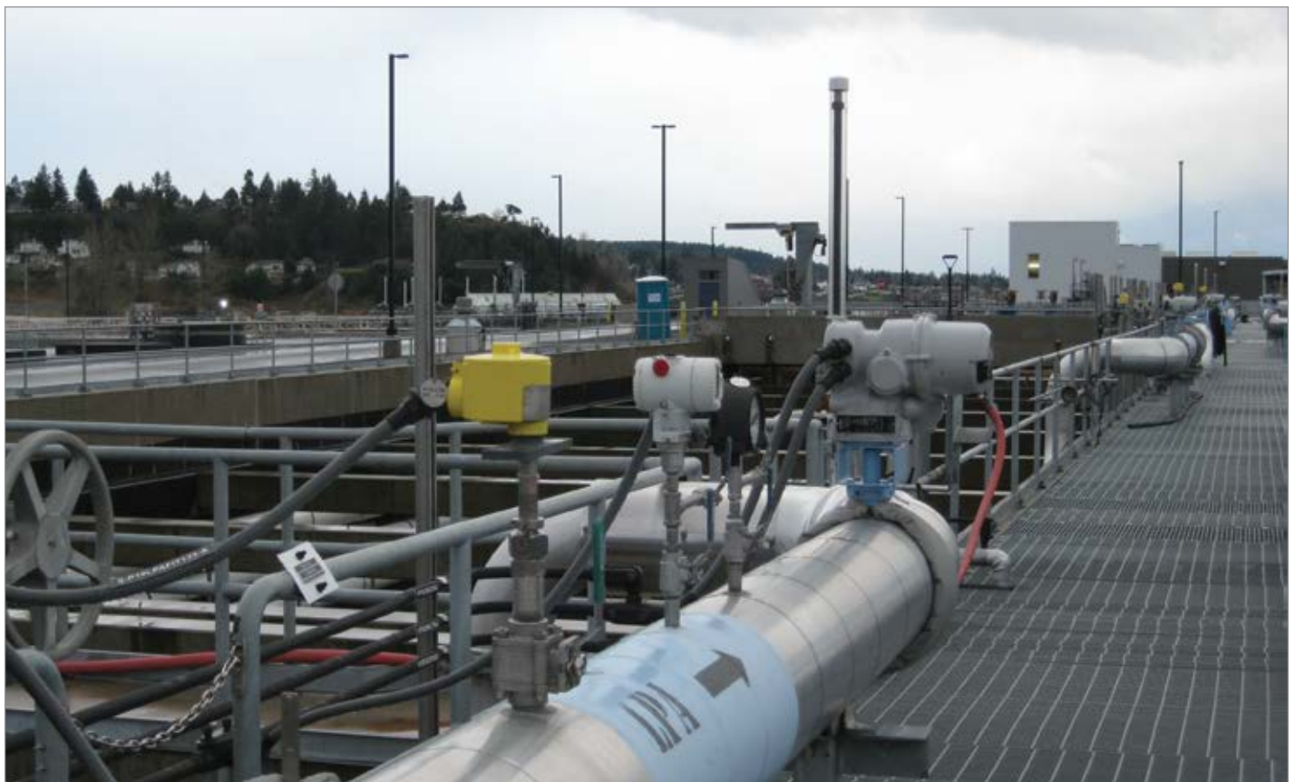
An algorithm is required to control the amount of air supplied to each aeration zone along the length of the basin.
