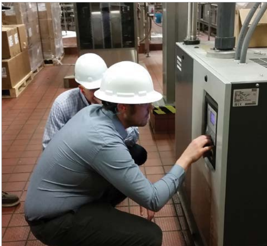
In addition to water savings, the Atlas Copco 350 GHS VSD+ rotary screw vacuum pump saves the brewery $4,000 per year in energy costs.
