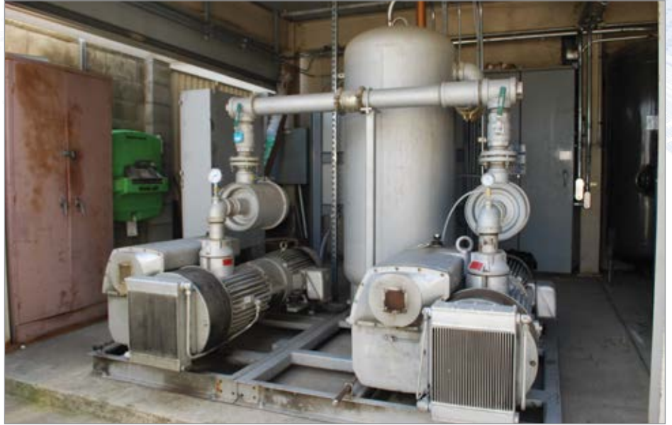
Shown are two 25 horsepower vacuum pumps used to move silicon wafers during the inspection process at the semiconductor plant.
