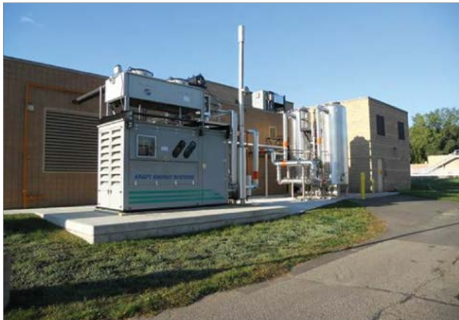
A number of Wisconsin wastewater treatment facilities leverage a host of technologies, such as this biogas-fueled generator set, to offset their energy consumption.
