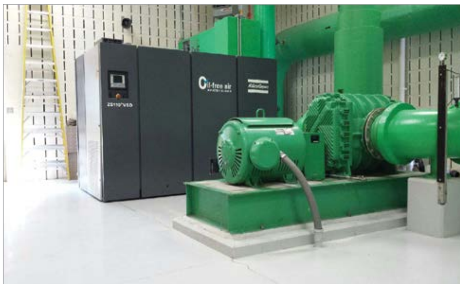
Shown is a rotary screw blower at a Wisconsin wastewater treatment facility.
