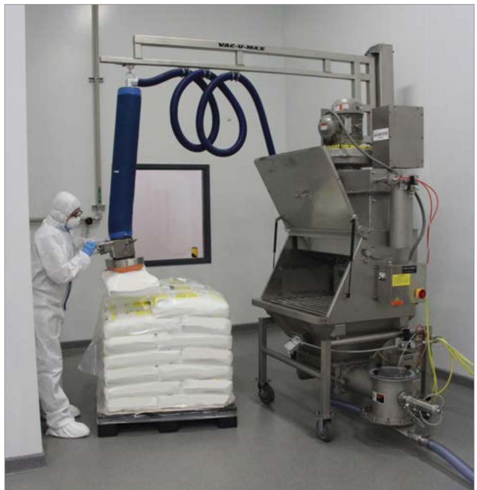
A bag dump station with integrated dust collection and load-lifter allows the operator to remove heavy bags from a pallet and easily place them on the bag station grate.
