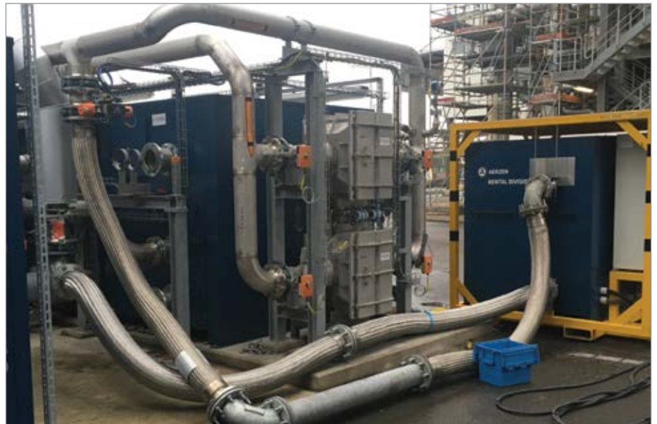
A rental blower helped a plant verify the benefits of a blower system upgrade.
