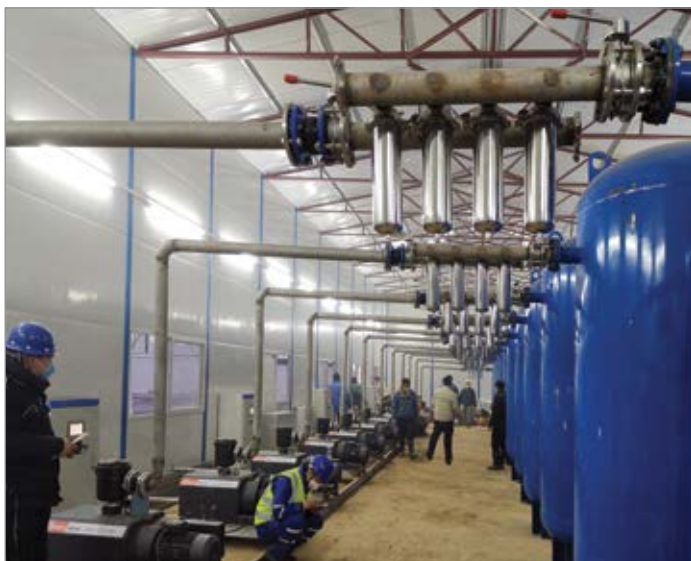
Vacuum pumps from Maulburg during the installation at Huoshenshan Hospital in Wuhan.
