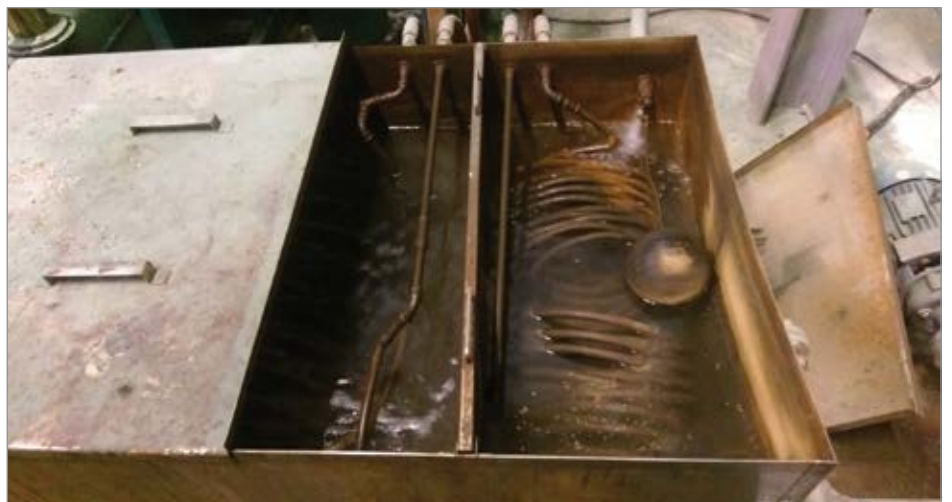
Figure 1: Existing System Sealant Reservoir and Cooler
