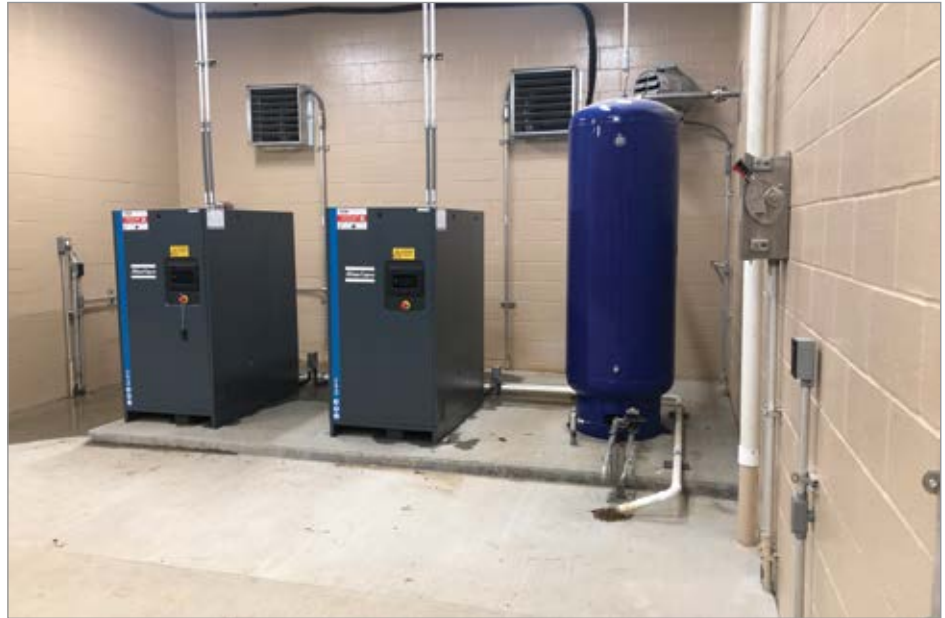
Air compressors provide high-pressure air for the compressed gas mixing system at the City of Highland's HWRF.
