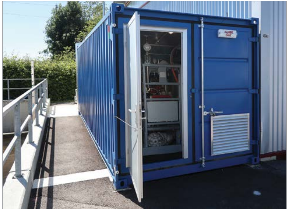
Figure 1. The new cogeneration unit at Echallens wastewater treatment plant is installed in a container. Using the biogas recovered from the sludge, it generates 150,000 kilowatt-hours of power per year.
