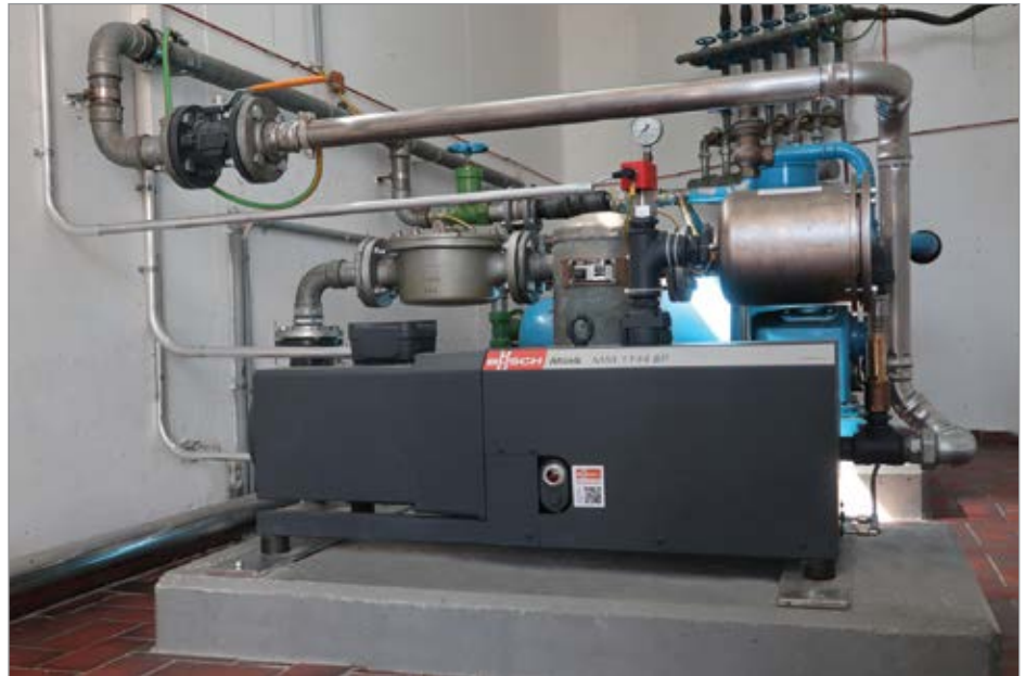
Figure 3. Up to 95 cubic meters of biogas per hour are transported by the MINK claw compressor at an overpressure of 0.6 bar.
