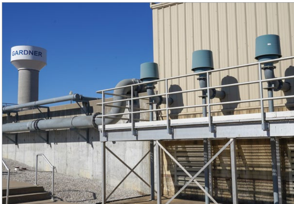
Existing intake filters and piping were reused, reducing installation costs for the new blowers.
