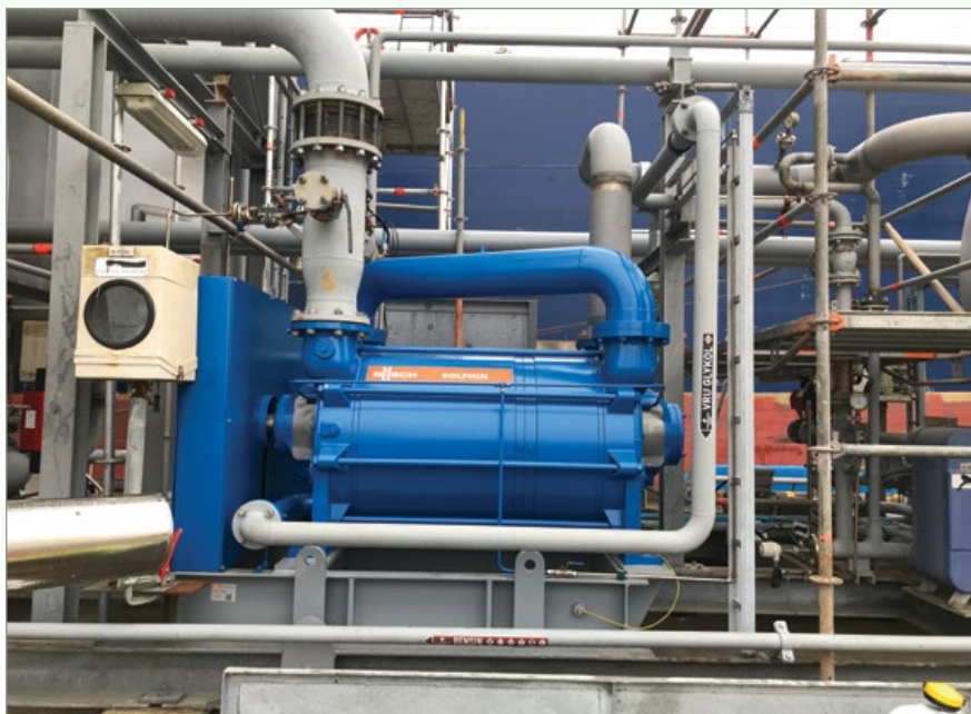
The tailor-made DOLPHIN liquid ring vacuum system solution installed in the vapor recovery unit at the Port of Gothenburg, Sweden. Source: Busch Sweden.
