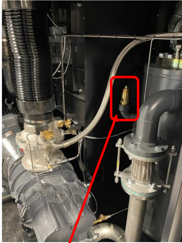
Tank Safety Relief Valve
